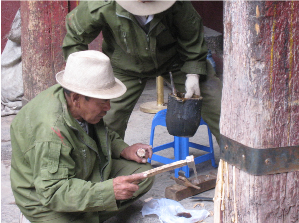
Inside the ancient Jokhang Temple, officials in charge of cultural preservation prefer to renovate existing structures rather than build new ones, wherever possible. Here, two Tibetan craftsmen repair a structural pillar more than 300 years old by hammering fresh wood into cracks and then shaping the wood to fit. (Jannuzi photo)
